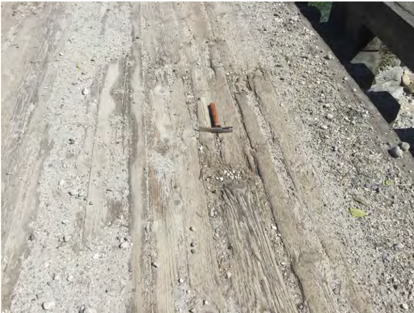
Span 2 Heavily Worn Deck
