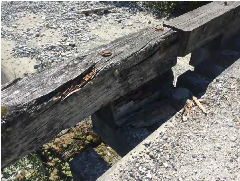
Rotten Guardrail and Riser
